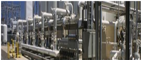
Longwatch Solutions Found in Energy and Utility Applications
