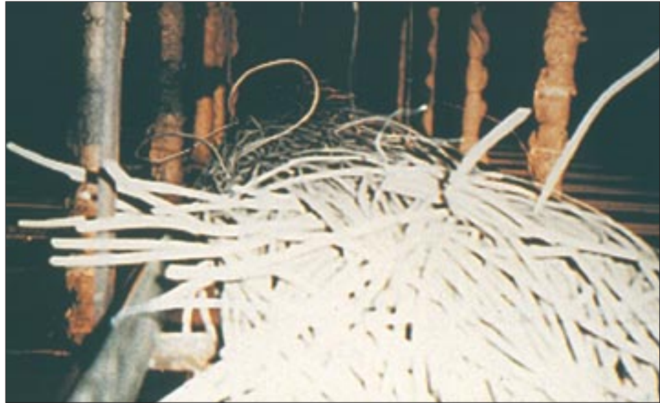
Figure 10 - Length of Cables on Ladder
