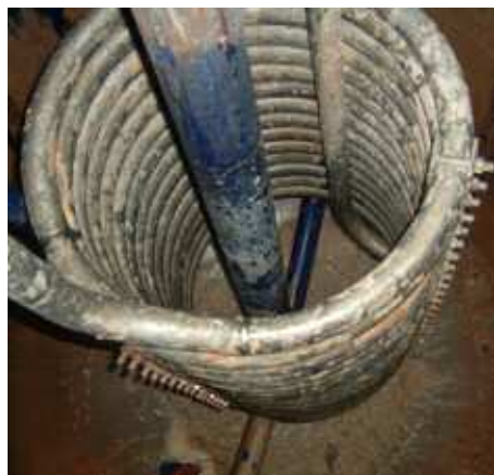
Changing dielectrics defeated old level devices. Note the tank's many internals.
