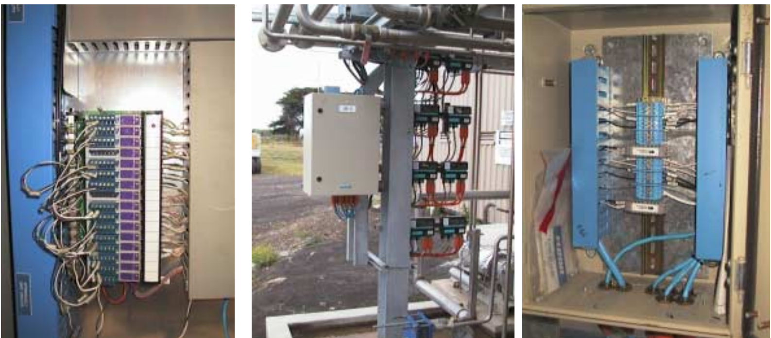
Figures 5,6,7: Barriers located in safe area (MTL 4053), Field cabinets, parallel field wiring with IS FF terminators (MTL)
