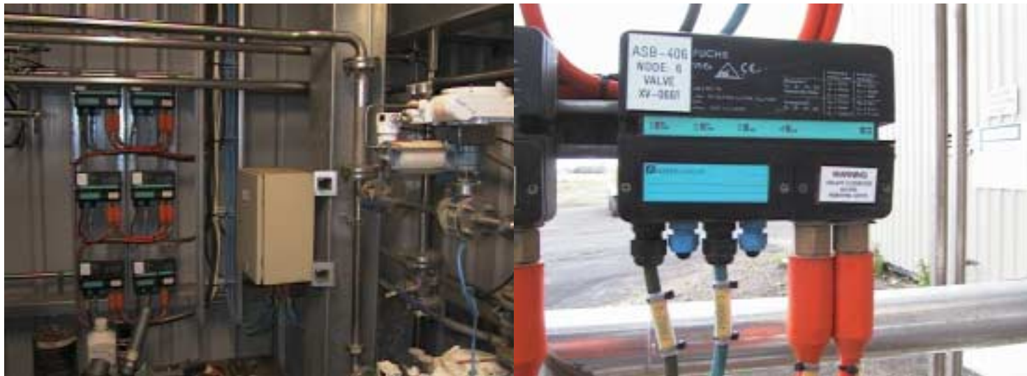
Figures 8 & 9: Asi slaves daisy chained together, individual module showing Asi Ex e wiring (right) and IS wiring (left) and individual LED indication.
