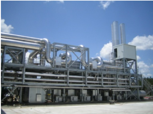
Fig. 2 -System manufactured by Dürr Environmental and Energy Systems.
